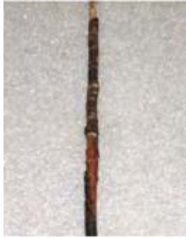
Worn Counterweight Cable
